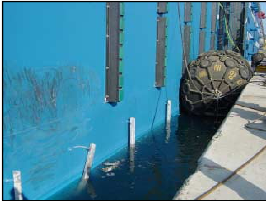
Figure 7. Anode damage resulting from contact with fenders during topside installation.
